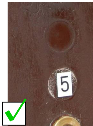
Fig. 11: OK Minor irregularities of surface and paint
